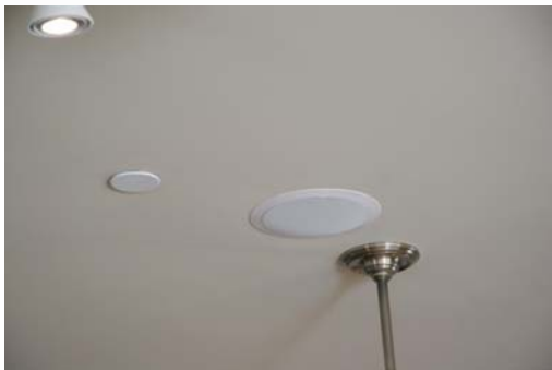
Flat Plate Concealed Fire Sprinklers like the one pictured above are less obtrusive than speakers and typical light fixtures
