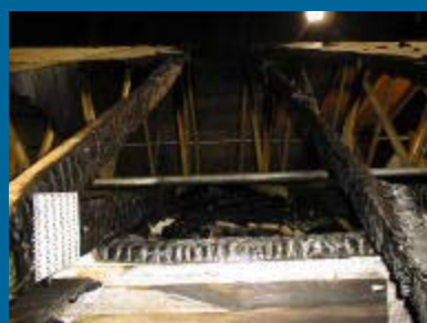
Damage Result of Task Group Acceptable Fire Test
